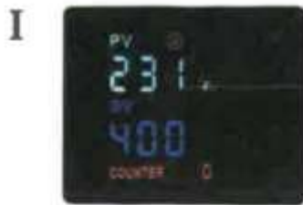
Control Panel Window
